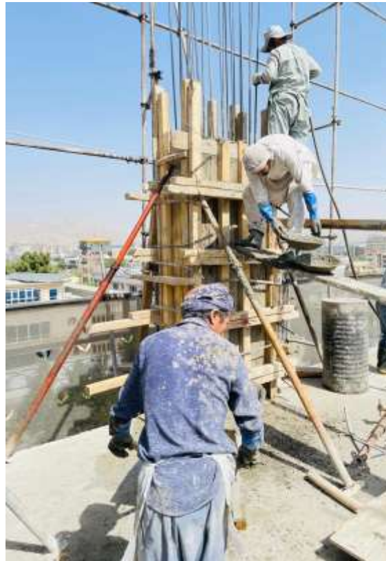
Figure 1 Field observation of unsafe work at height during concrete casting in Kabul, used as evidence in the FMEA process.
