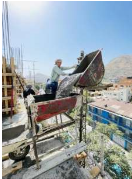
Figure 4: Unsafe rooftop lifting operation, where workers stand close to suspended loads without proper safety distance.
