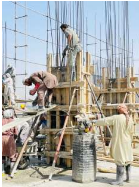
Figure 3: Unsafe scaffolding work at height without proper fall protection
